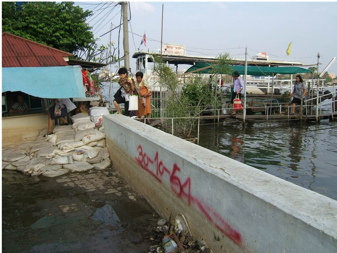
Photo: Discontinuous dyke caused of flood in Bangplatt district/ Credit: Rumana Kabir, UNDP
